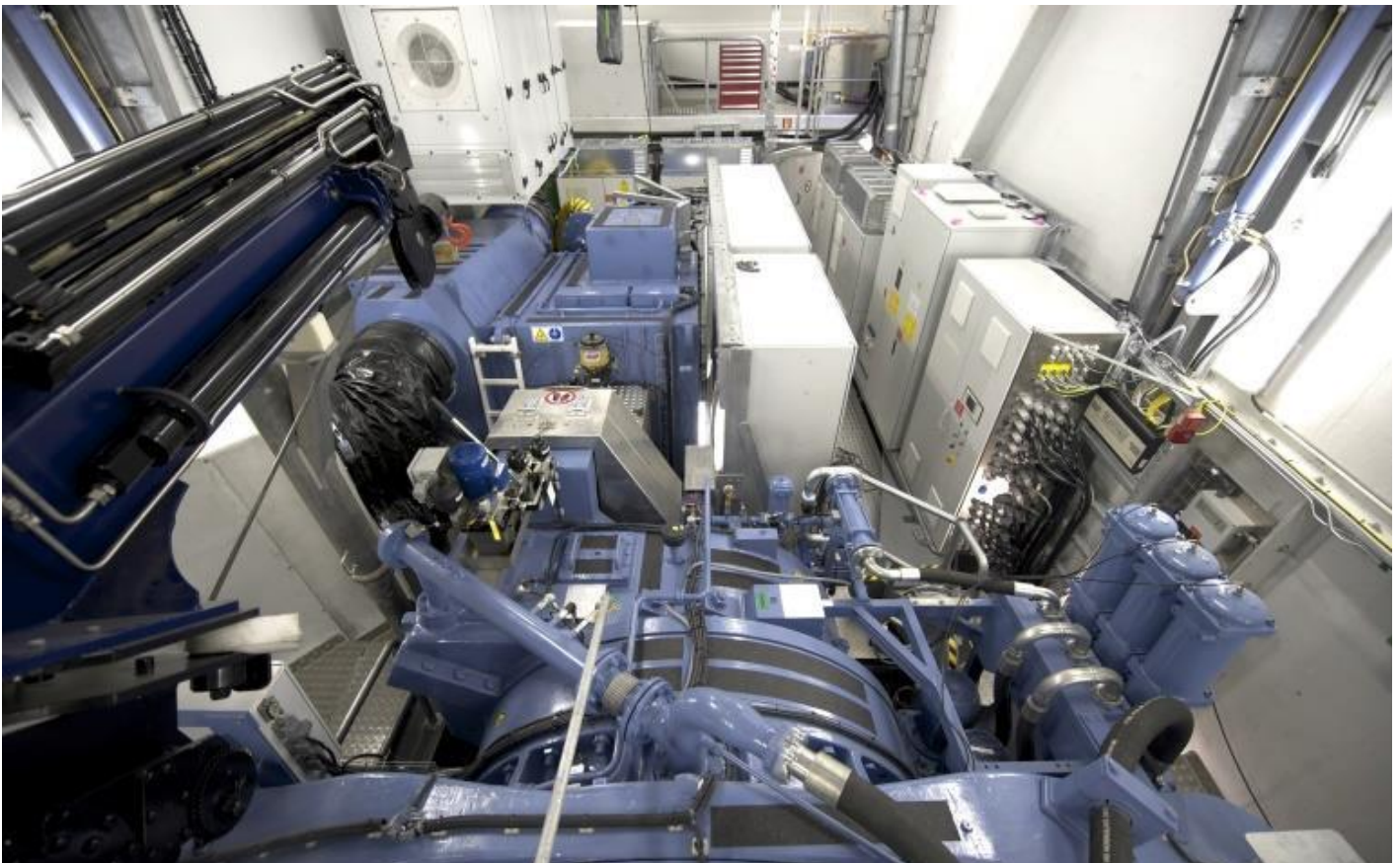
Drivetrain inside the hub of a wind energy system
